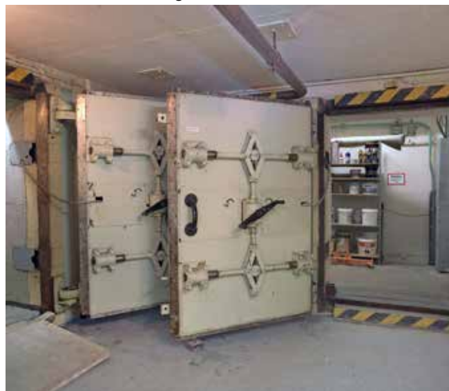
The entrance blast doors at Wollenberg. The door on the right goes straight into the bunker, that to the left goes through the decontamination area. Photo Nick Catford
